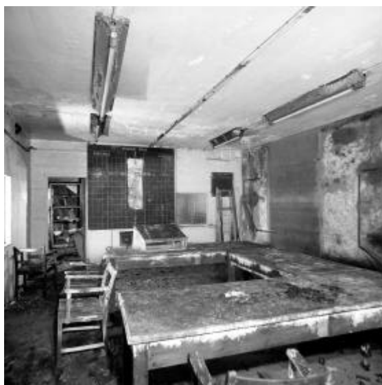
The control room
